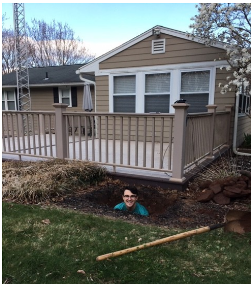
K1LYP'S GRANDSON DIGGING THE NEW TOWER BASE AT THE LYP TOWER FARM
